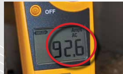
Amp measurement without 5-2-1 ® Compressor Saver ®
